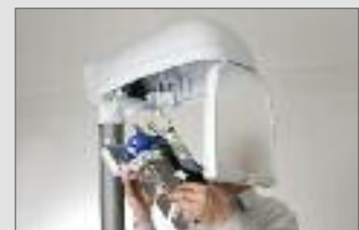
6. Remove the gear tray and replace with a new LED generation gear tray.
